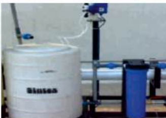
Chemical Dosing System
