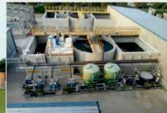
Effluent Treatment Plant ZLD
