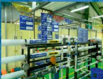
RO Recycle Plant
